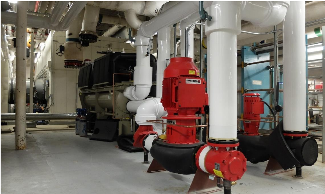
Heat recovery chiller and pumps installed at Vancouver General Hospital.
