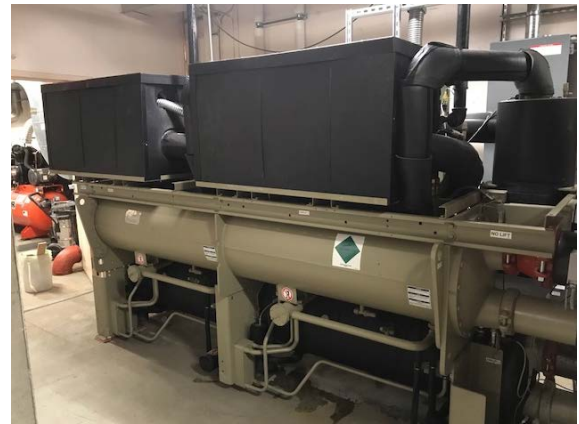
Figure 1: New Heat Recovery Chiller
