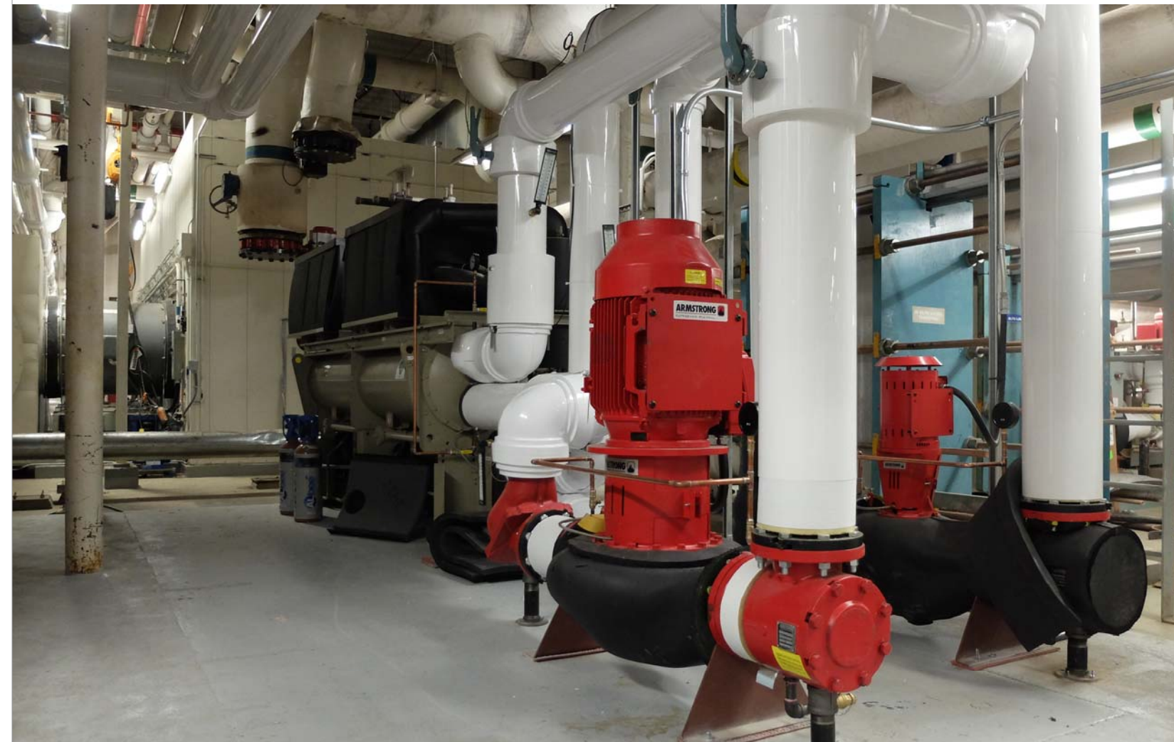
Figure 3: Heat recovery chiller and pumps installed at Vancouver General Hospital.
