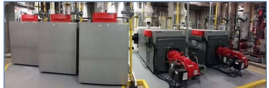
Powell River General Hospital: Energy efficiency upgrade.
